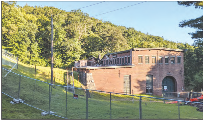
A full shot of the Red Bridge Hydro Plant on 5 Red Bridge Rd. which experienced a building collapse and small fire on Aug. 22.
